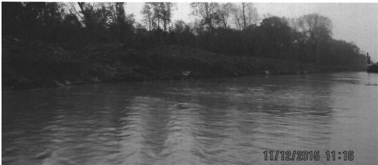
Fig.9: Picture taken on 11/12/2015 of construction on the Buffalo Cove Water Management Unit Project
