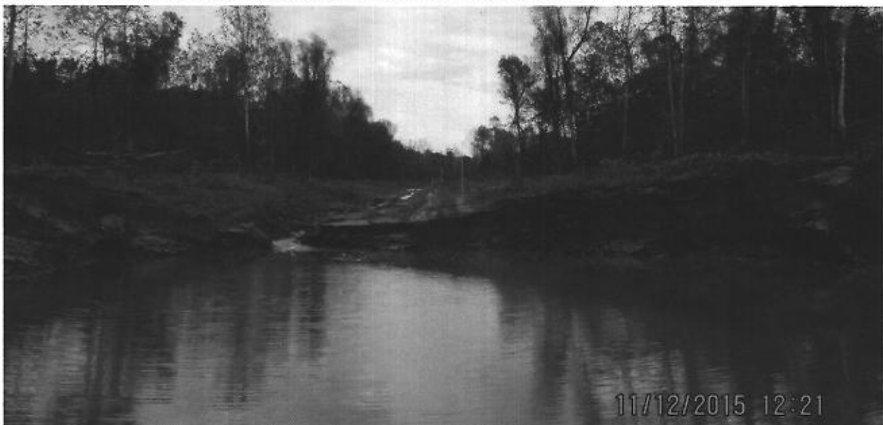
Fig. 10: Picture taken on 11/12/2015 of construction on the Buffalo Cove Water Management Unit Project
